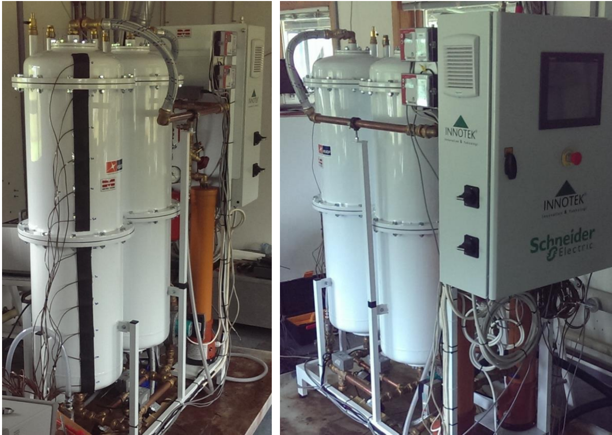
Figure 15 - Storage tank test setup with two storage tanks, an electric resistance heater and control system. The row of thermocouples is shown mounted on the storage tank.
