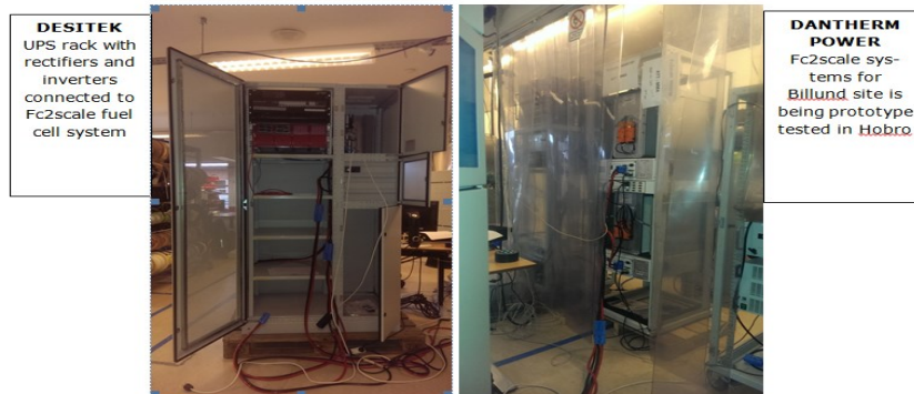
Figure 29 Field system setup tested in lab before its installed at Billund site. At the left UPS rack from Desitek, and at the right the fuel cell system.
