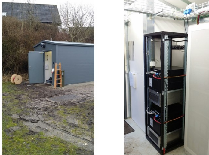
Figure 32 Løgstør system site with 2x1,7kW fuel cell systems installed in a Intego shelter with integrated H2 bottle room.
