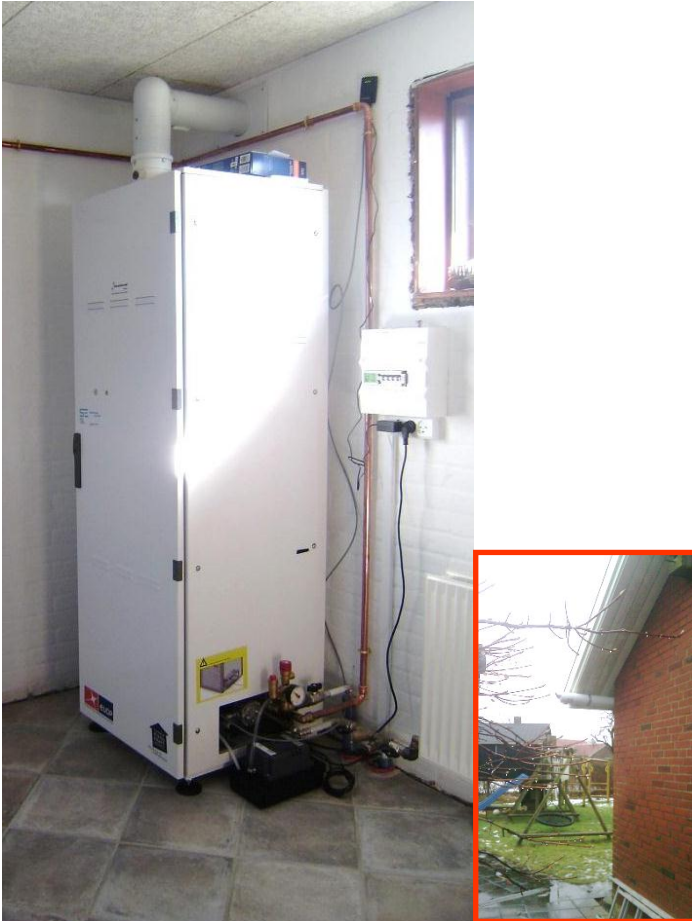
Figure 26: One of 20 fuel cell mCHP systems installed in the field
