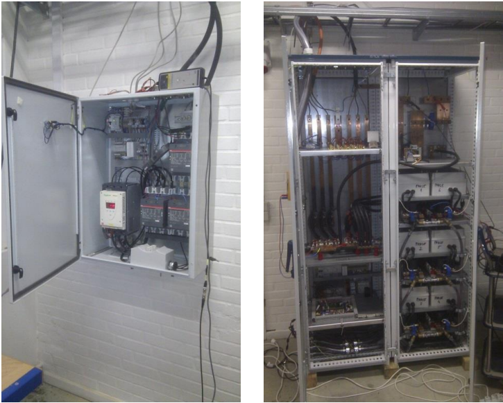
Fig. 5.3. Pictures of the simple prototype installed at GH.
