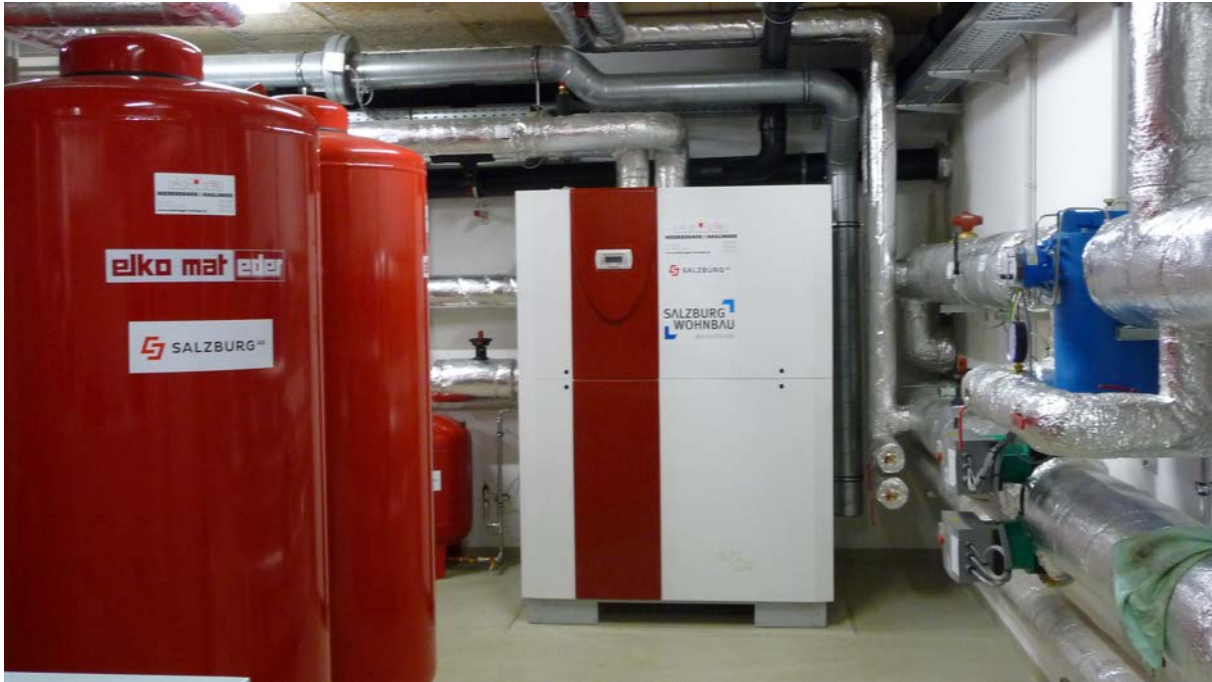
Figure 17: Central energy station of the residential building complex
