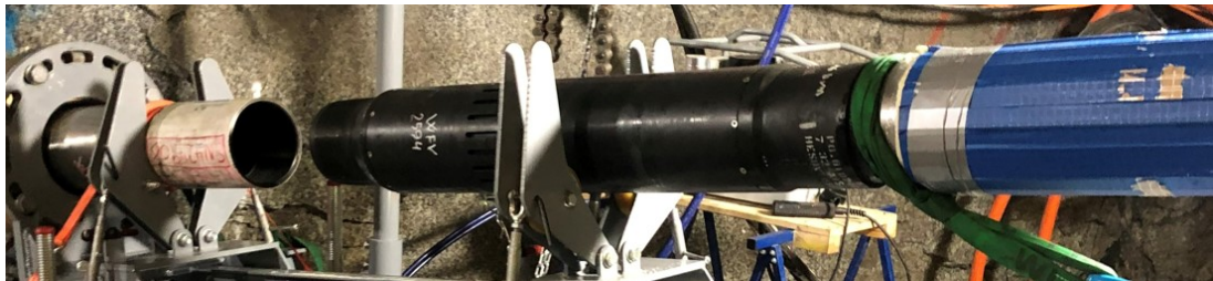
Above: A picture from Bedretto, where a flow valve, already connected to a packer, temporarily wrapped in blue packaging is about to be connected to a 7" pup-joint with a packer already partially in the well.
