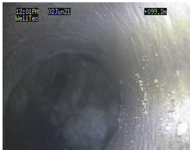
Above: A screenshot from a camera of the originally 120-meter-long test borehole blocked at 99 meters.
