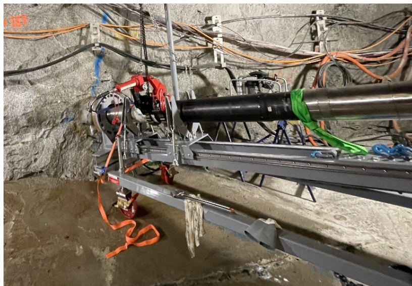
Above: Flow valve (black, left) and packer (right) installation in Bedretto (August 2021)
