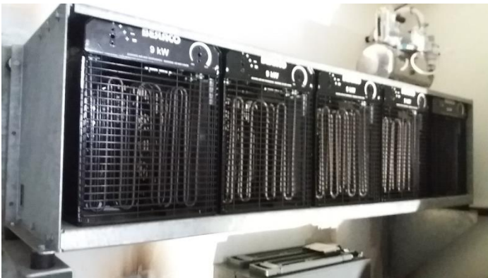
Figure 2. Photograph of the five 9 kW dumploads installed on the Tordenskiold.
