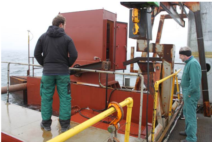
Figure 2. The (same) PTO system on the P37 platform during offshore testing.
