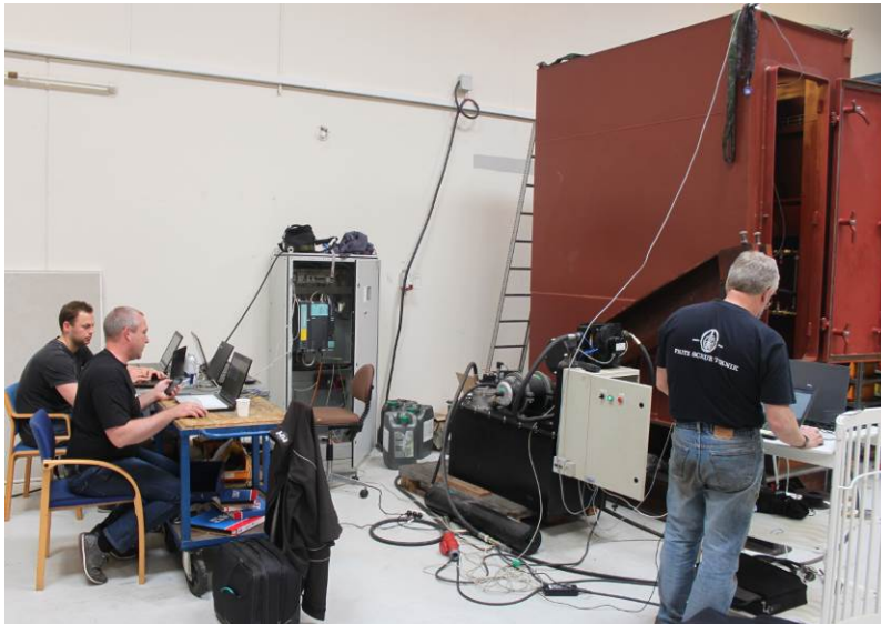
Figure 1. The P37 PTO system during dry testing between offshore tests.
